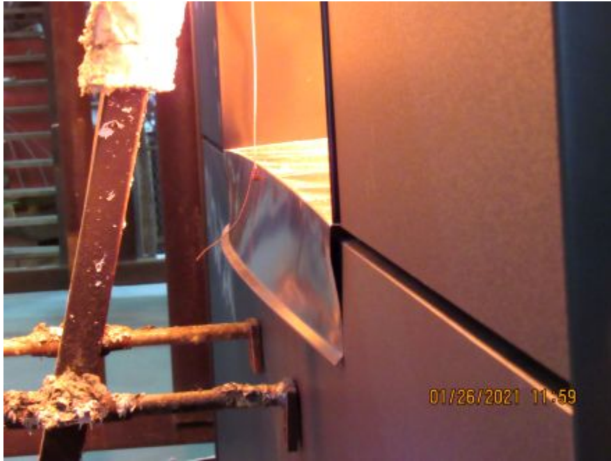
Photo No. 27 Window sill flashing warped
